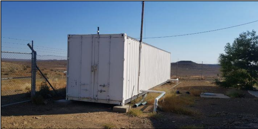
FIGURE 4: RO & UF PLANT
