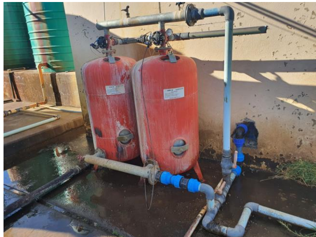
WTW Sand Filters
