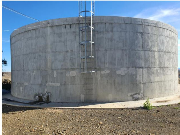
Potable water Reservoir
