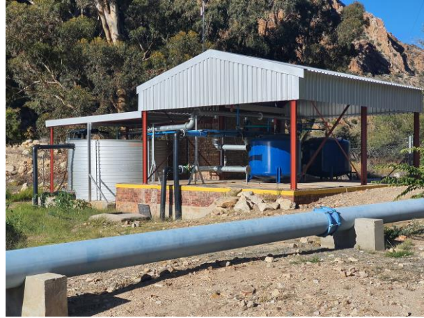
Iron Removal Plant
