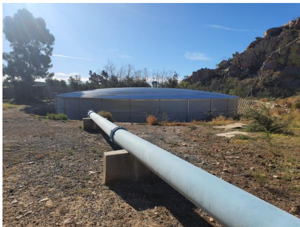
Storage Reservoir @ WTW
