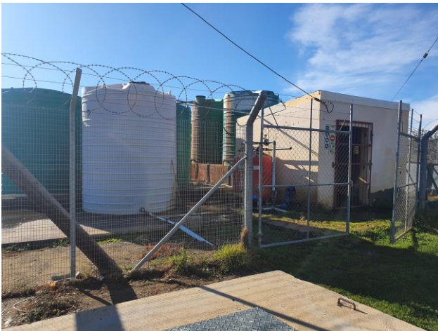
Water Treatment Works
